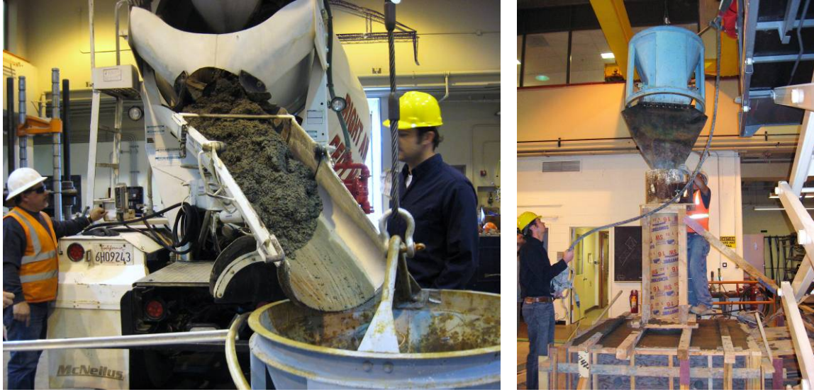
Figure B-10 (a) Fiber-reinforced concrete mix poured to concrete bucket; (b) Casting of fiber-reinforced concrete columns
