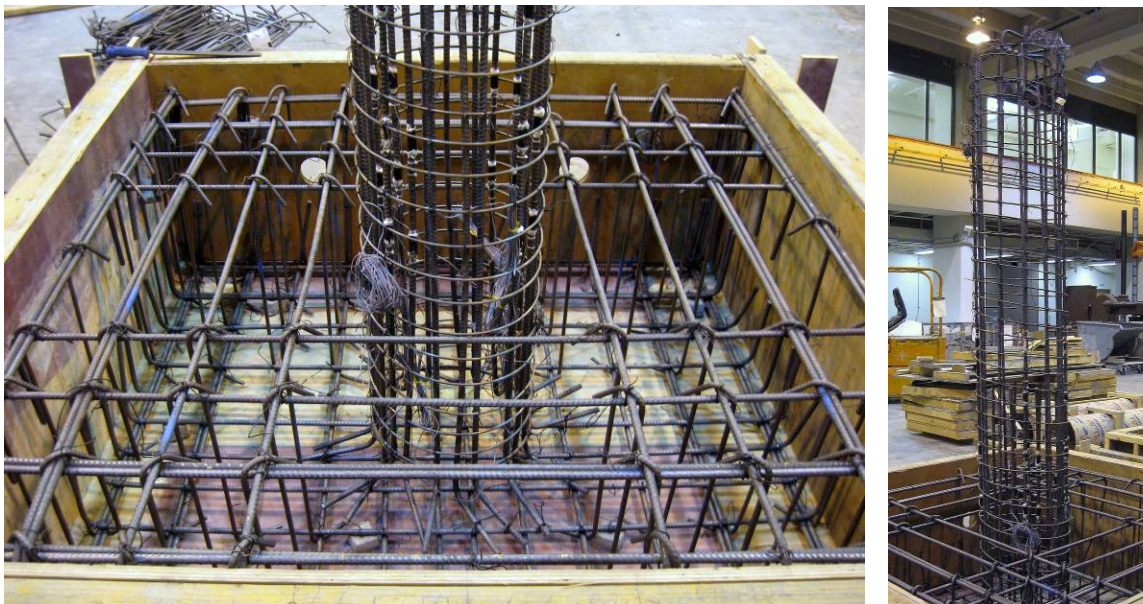
Figure B-1 (a) Anchor block formwork and unfinished cage; (b) Column cage
