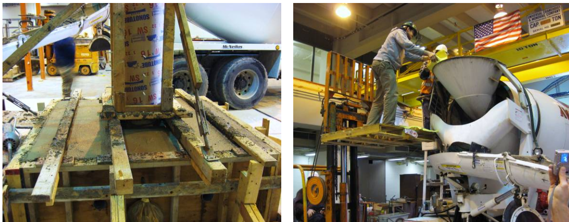
Figure B-9 (a) Finished surface of anchor block; (b) Fibers added to concrete mix inside truck
