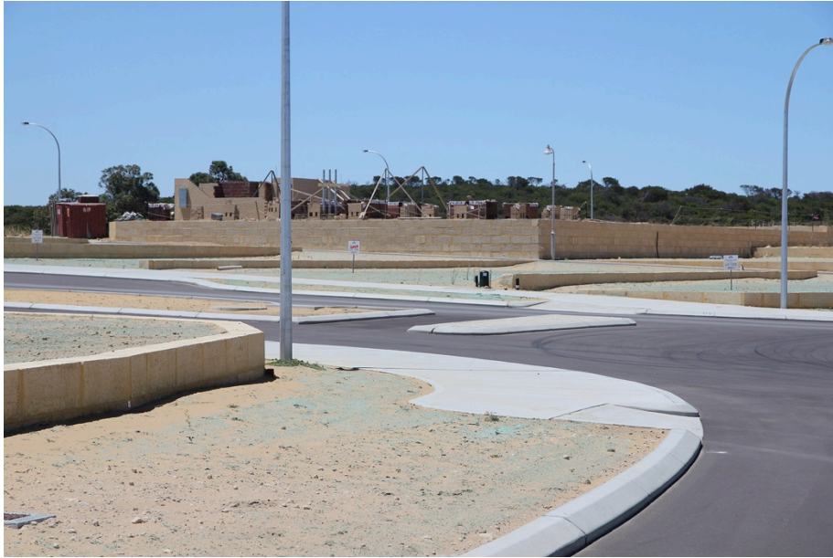
Figure 21: ground-level view at Capricorn through empty terraced lots. House under construction in background is setback the minimum 1m distance from retaining walls on lot boundary (author 2012).
