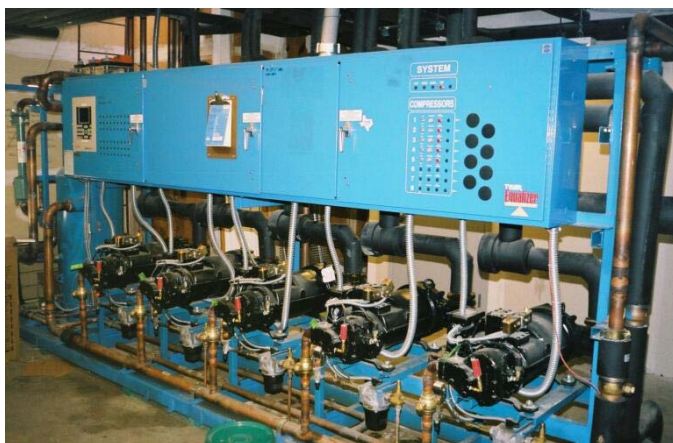
Figure A- 25: Compressors Inside of Control Room
