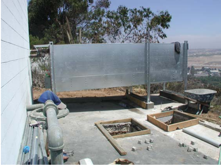
Figure A- 34: Site for the Two 150 kW Natural Gas Engines with Excess Heat Radiator in Background
