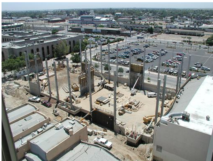
Figure A- 27: Construction of Parking Garage Where Fuel Cells Will Be Housed
