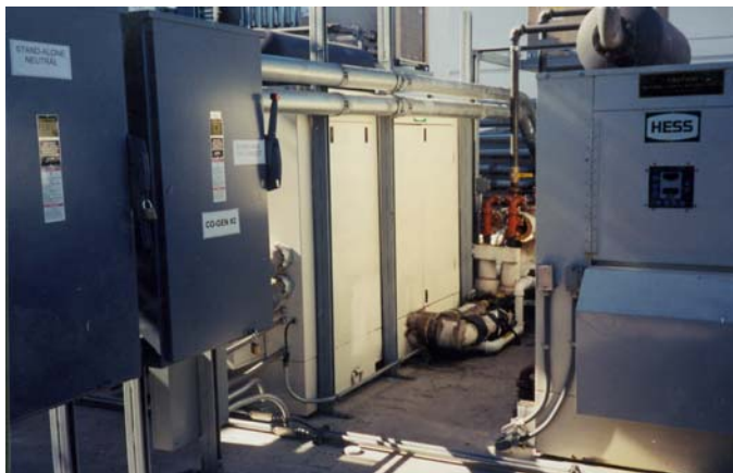
Figure A- 30: Generation Equipment (Propane Engines) and Islanding Switch
