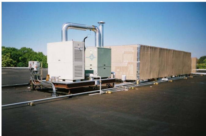
Figure A- 24: Capstone 60 kW Microturbine, MicroGen Heat Exchanger, and Munters Unit
