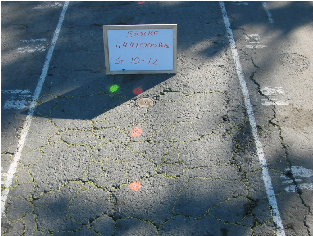
Figure 3.28: Surface cracks marked with crayon between Stations 10 and 12 at end of test.
