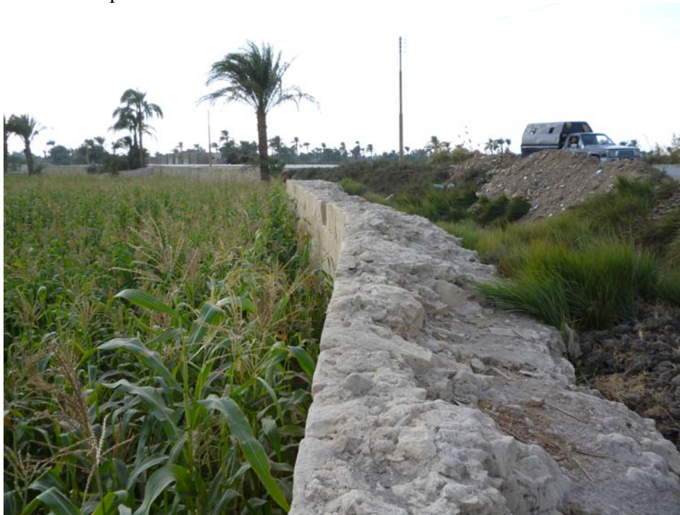
Fig. 18: A masonry-faced section of the dam near the village of Iṣṣā. Photo: B. Haug, November 18, 2011
