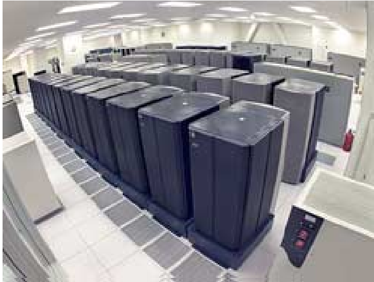
DATA CENTER FACILITY 5
