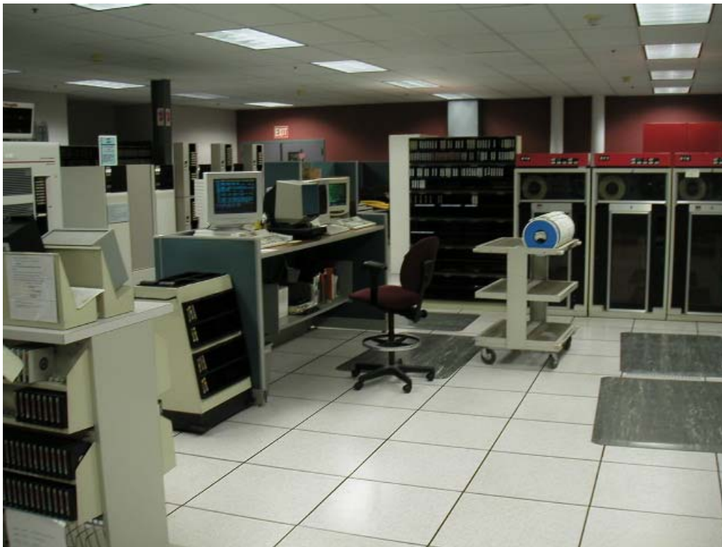
Figure 5. Main Computer Room
