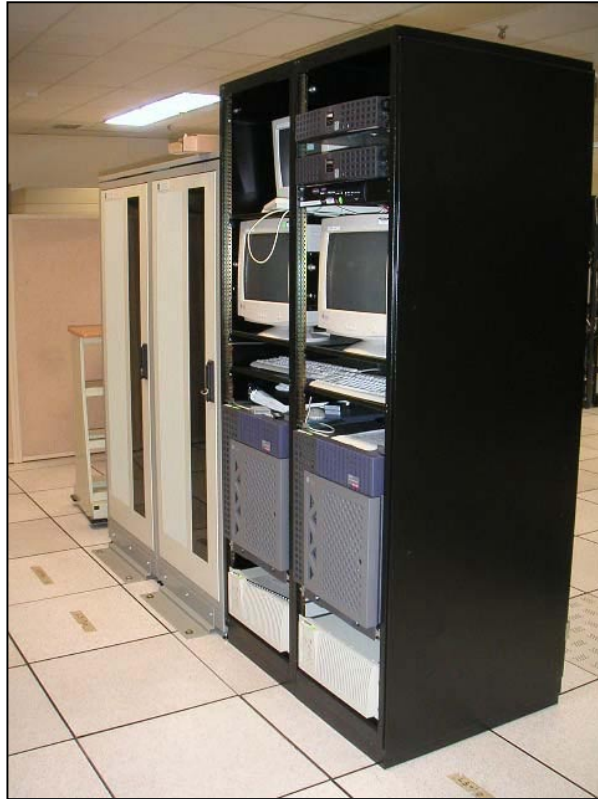
Figure 6. Servers in Data Center 4.1
