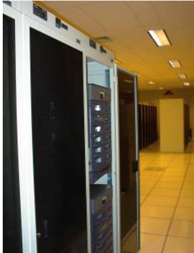
Figure 7 Server Cabinets and Racks
