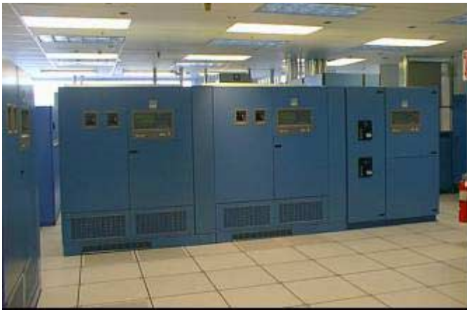
Figure 10 An older UPS system
