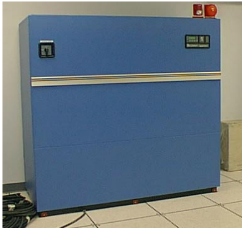
Data Center CRAC Unit
