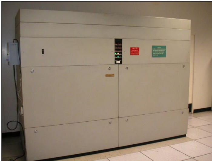
Figure 9. CRAC 7 in Data Center 4.1
