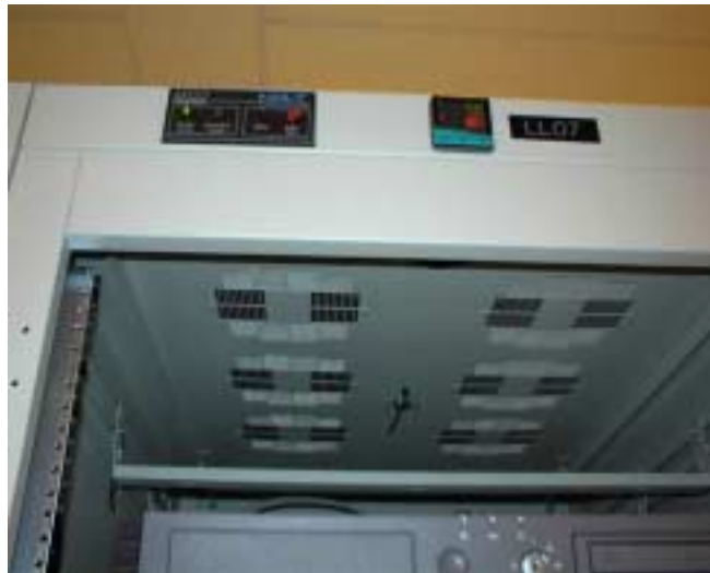
Figure 7 Top of cabinet showing fans
