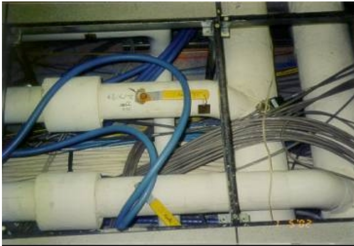
Figure 14 This under floor area in the NY Data Center severely restricts air flow
