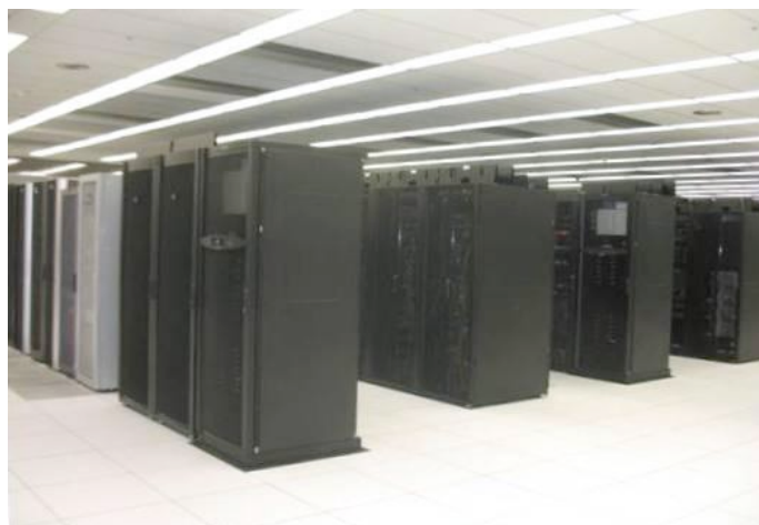
Figure 2-1: Demonstration Data Center IT Equipment
