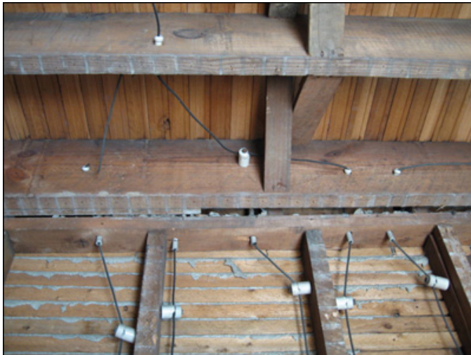
KNOB AND TUBE WIRING IN A WALL AND CEILING
