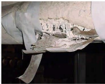
Friable asbestos pipe insulation
