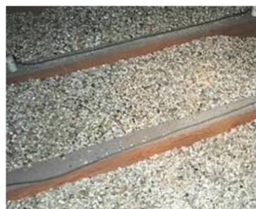
Asbestos-containing vermiculite attic insulation
