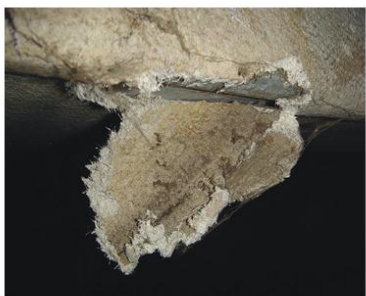
Detail of friable asbestos duct insulation
