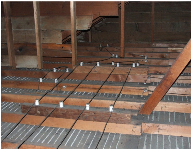
KNOB AND TUBE WIRING IN AN ATTIC
