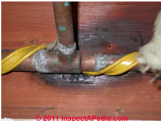
© 2011 InspectAPedia.com HEAT TAPE AROUND PIPE (CHARRING LIKELY CAUSED BY BRAZING)
