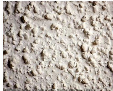
Detail of asbestos textured ("popcorn") ceiling
