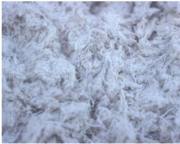
Asbestos loose-fill insulation (rare in residential buildings)
