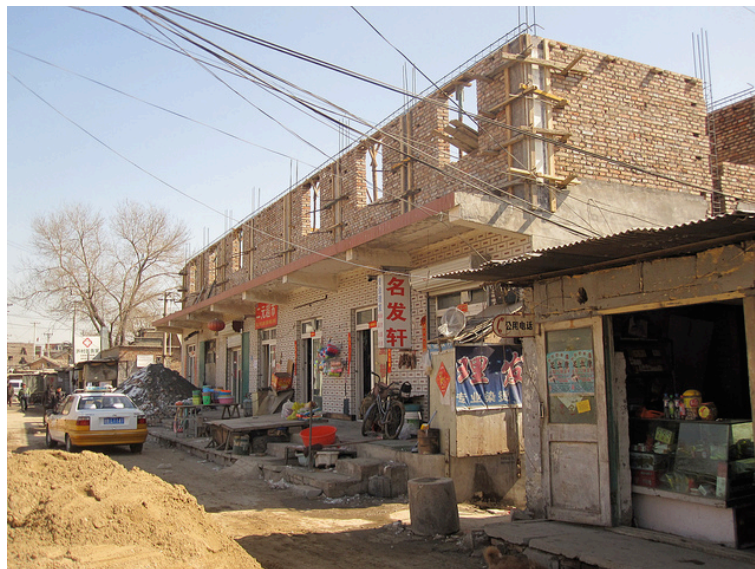
Figure 2.3 An extra floor being constructed on top of an existing building. (Dongxiaokou Village, Changping District; March 9, 2010)
