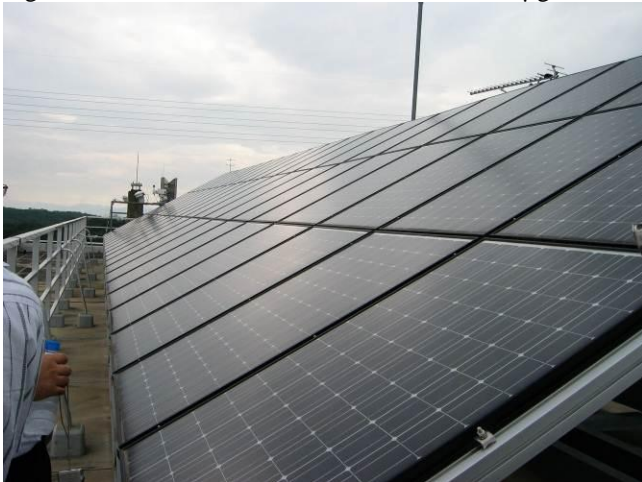
Fig. 4. PV array in the AIT DC \mu grid
