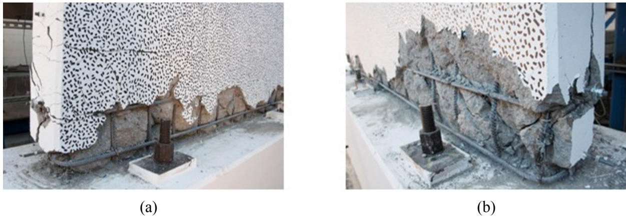
Figure 6.49: Wall 2 Final Damage State after Removing Broken Concrete: (a) East Side (b) West Side
