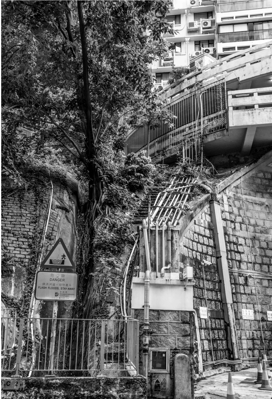
Exposed utilities infrastructure. Registered slope 11SW-A / CR19. [Karl Kullmann]
