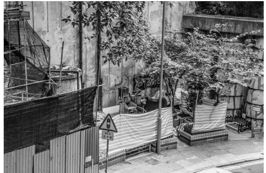
Public plaza used for temporary storage during maintenance on registered slope 11SW-B / C65. [Karl Kullmann]
