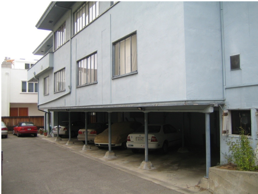
Figure 1. Photo of an example soft-story property in Berkeley.
