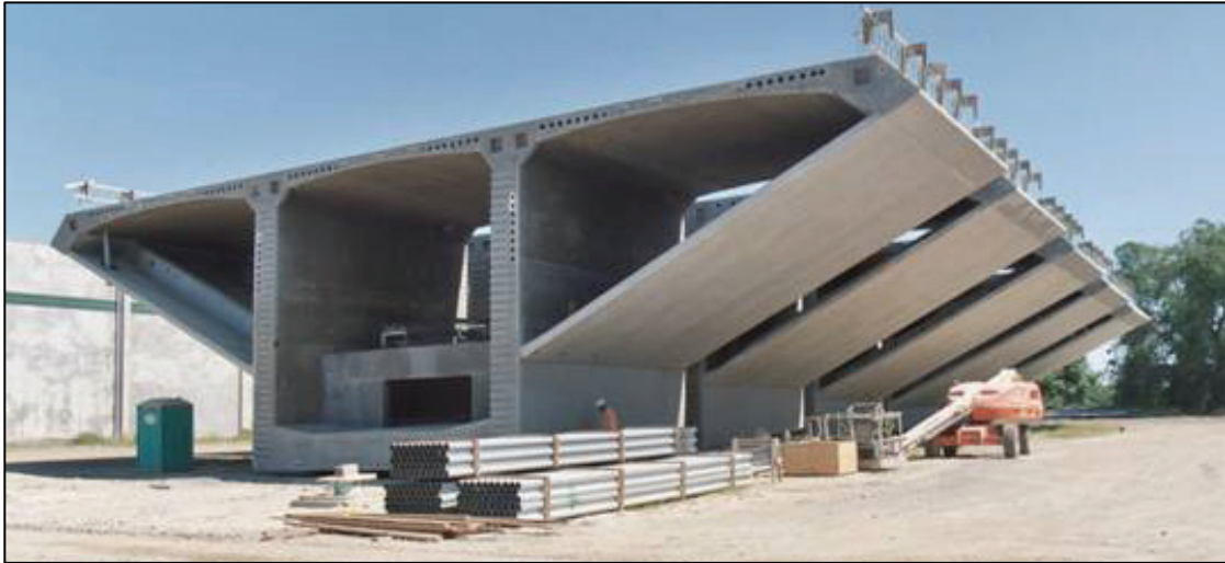
Figure 2-2 Precast Superstructure Segments for the San Francisco-Oakland Bay Bridge Skyway in the Stockton Casting Yard ready for Transport by Barge to the Bridge Site
