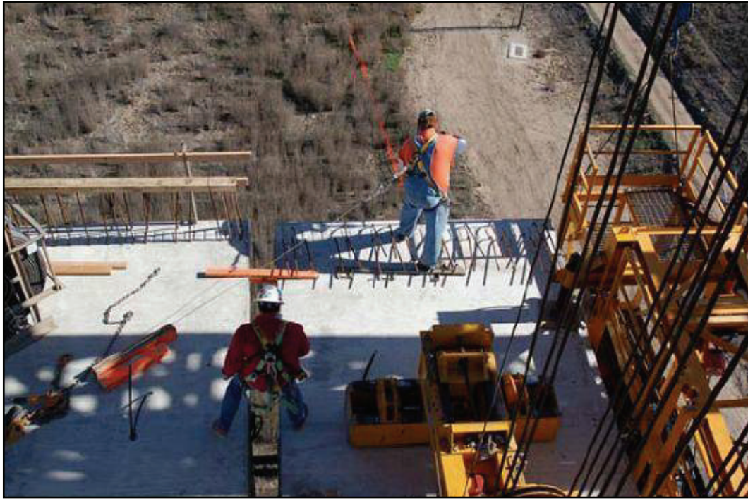
Figure A-13-49 Otay River Bridge - Segment Installation (Courtesy of International Bridge Technologies)
