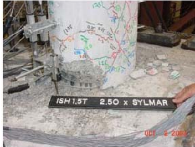
Figure 2.5- Damage state DS-5, imminent failure, cracking inside concrete core.
