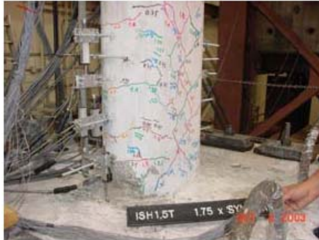
Figure 2.3- Damage state DS-3, extensive cracking and spalling.
