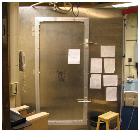
Figure 4.11. Photograph of the second generation shielded room, installed in Birge B203.
