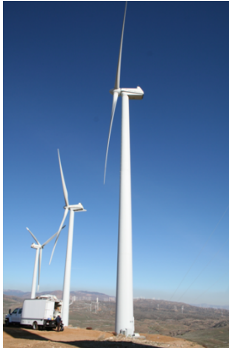
Figure 2.1: Tested wind turbine provided courtesy of Oak Creek Energy Systems (photo courtesy of Prowell, 2010b).
