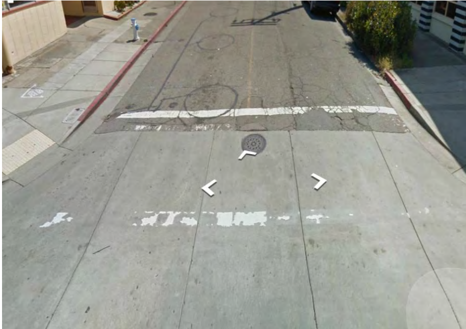
Figure 33. Example of “Faded” Crosswalk Condition
