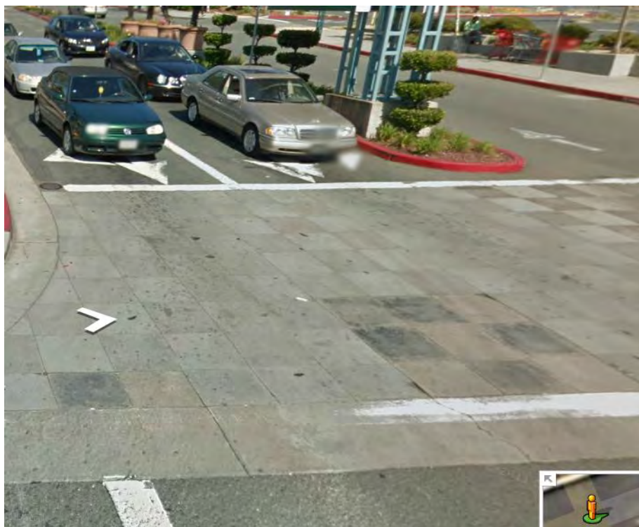
Figure 32. Example of “Partially Worn” Crosswalk Condition
