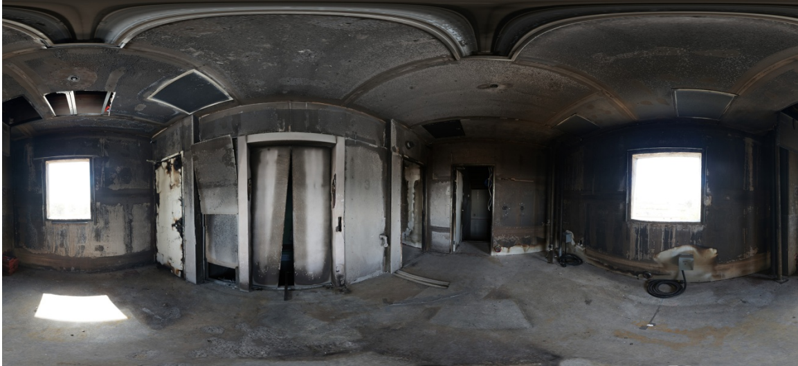
Figure 1.7 Spherical panorama of the third floor after earthquake and fire test sequences.
