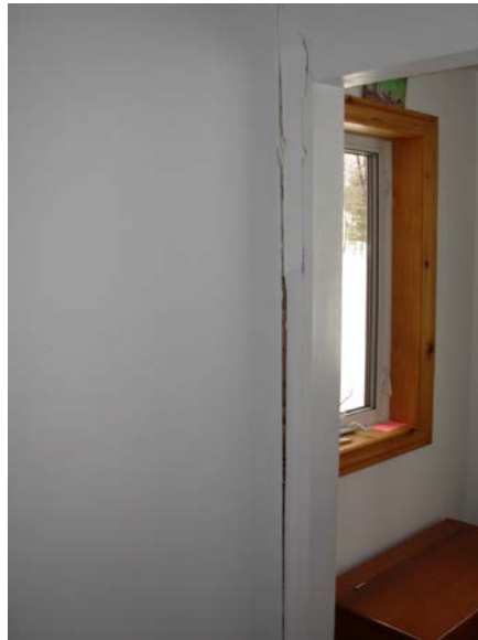
Figure 1.9 2010 Eureka California ( M_w=6.5 ): interior PW damage. (From Eureka Earthquake Clearinghouse, 2010)
