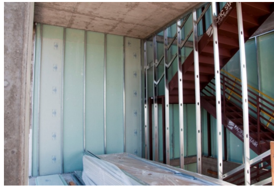
Figure 1.6 Overview of PW installation within the BNCS project.
