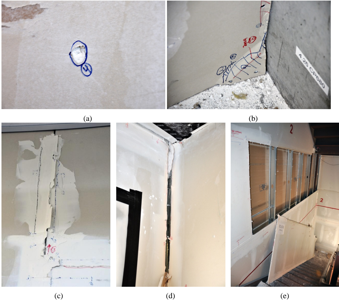
Figure 1.8 Typical PW failure modes observed during the BNCS test project at UCSD: (a) screw pull-through, (b) crushing in corner and along return wall, (c) tape flaking/cracks along panel boundaries, (d) gap and damage concentrated at intersection of wall boundary, and (e) detachment of panel.
