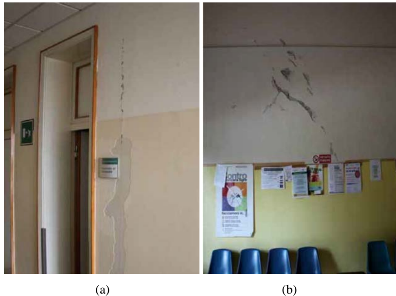
Figure 1.15 2012 Emilia Earthquakes ( M_w=6.1 ): interior PW damage within a hospital in Bondeno, Italy. (From Magenes et al., 2012)
