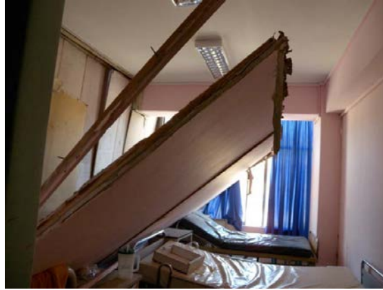
Figure 1.10 2010 Maule (Chile) Earthquake ( M_w = 8.8 ): interior PW damage from Felix Bulnes Hospital in Santiago demonstrating a collapsed out-of-plane wall. (Photo from: G. Mosqueda)
