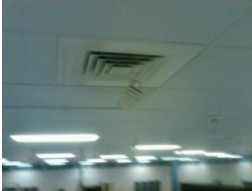
Figure 9 - Typical Coupon Mounting, Example Shown at Data Center Room Supply or Return Grill
