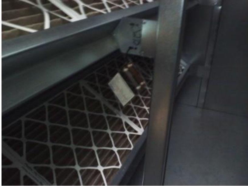
Figure 7 - Typical Coupon Mounting - Example Shown is Immediately Downstream of Supply Air Filters as Found in Large Roof Top Fan Units
