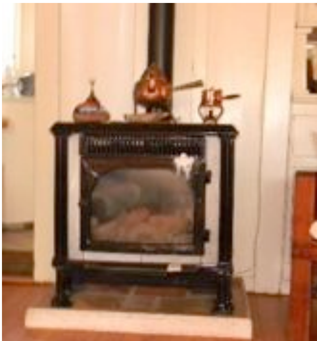
Figure 3.9 A picture of the gas fireplace at Site 1405, which has been identified as the cause for the elevated CO levels measured at the home.
