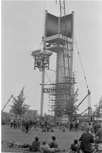
Figure 6. Locals watch as the bells of the Philips Carillon are lifted by crane into the belfry.
