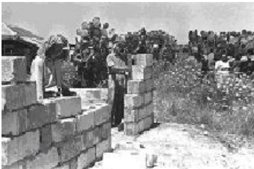
Fig. 6.21 Immigrants from Sophia, Bulgaria, building an additional structure for their family now living in one room in Azur. June 1949.
