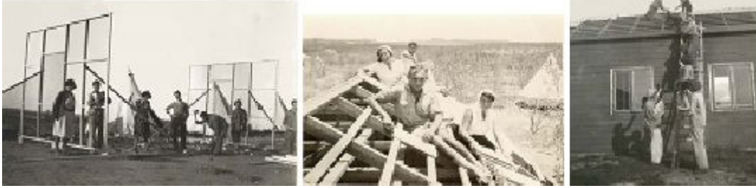
Fig. 5.20, 5.21, 5.22, Construction of wooden shacks by the Beit Alpha members from disassembled parts. Source: Beit Alpha archive.
