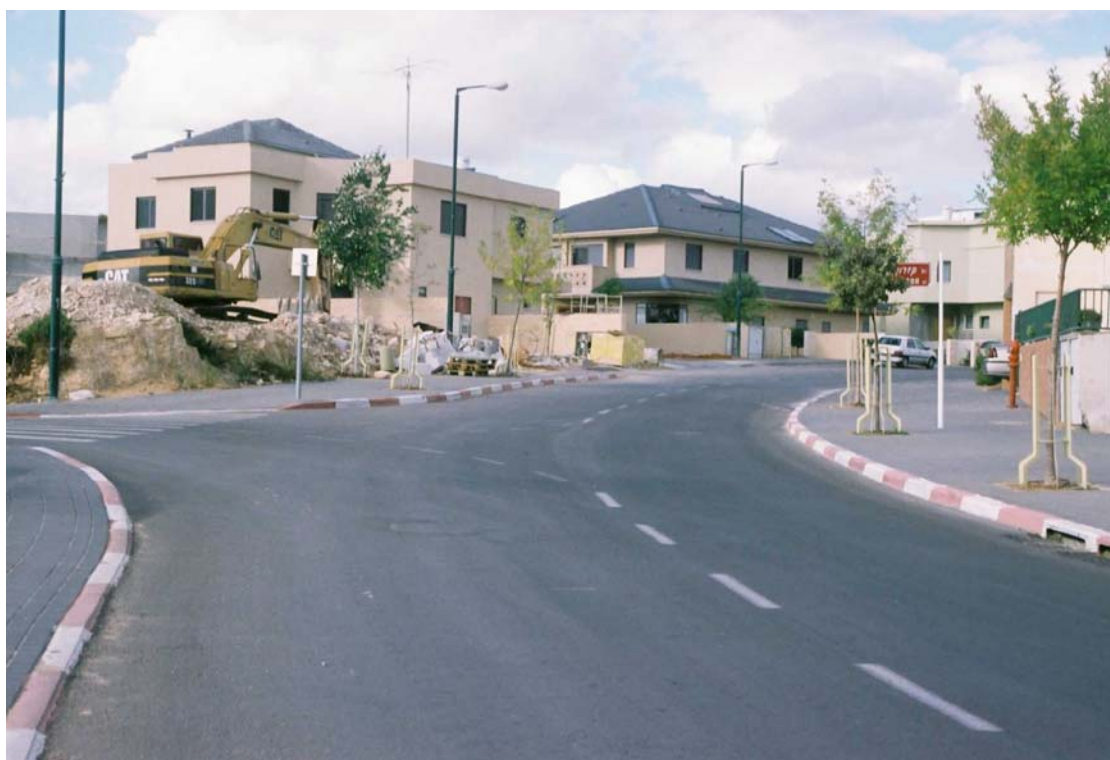
Excavator parked next to a new home being built in Alfei Menashe Photograph by Yael Warshel
