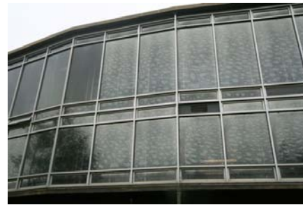
Failed window film treatment.
