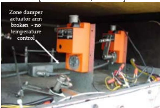
Zone damper actuator arm broken (no temperature control) [Martha Hewett, MNCEE]
