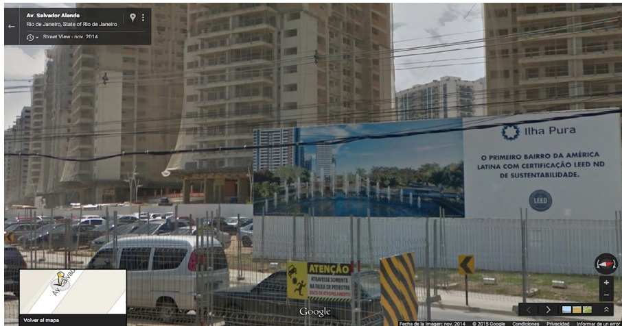
Figure 9. The construction of the Olympic Village, Ilha Pura, and a billboard with the following notice in Portuguese: Ilha Pura: The First Neighborhood in Latin America with the LEED ND Certification of Sustainability. Rio de Janeiro, November 2014, Google Street View https://goo.gl/maps/T2AL7 .
