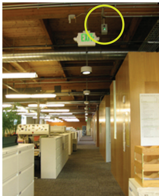
Red/green signals are located overhead in corridors, with other utilities
