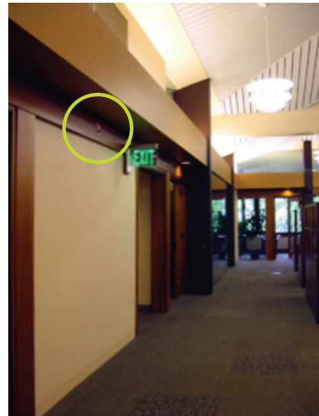
Signals are installed in the circulation areas between perimeter and core offices
