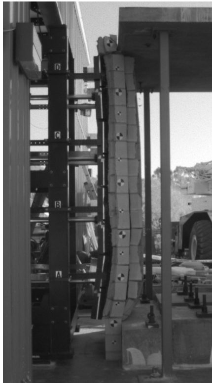
Figure 6.24: Test 1- BGs punch through wall
