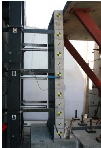
Figure 4.23: Test 5- CMU 3 post test
