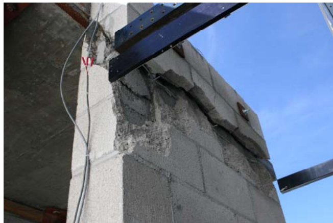
Figure 4.18: Test 3- CMU 1 shear failure post test
