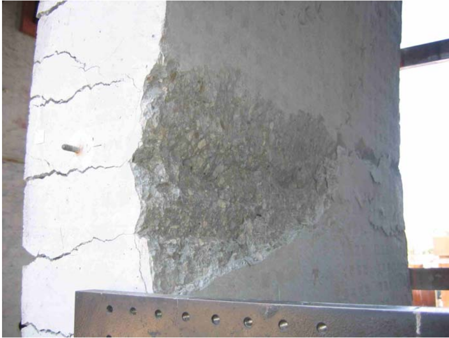
Figure 5.22: Series I Test 6- Damage to compression concrete
