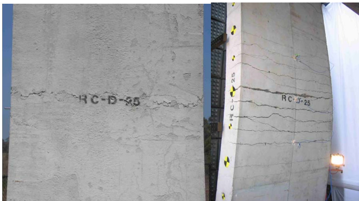
Figure 5.21: Series I Test 4- Post test damage
