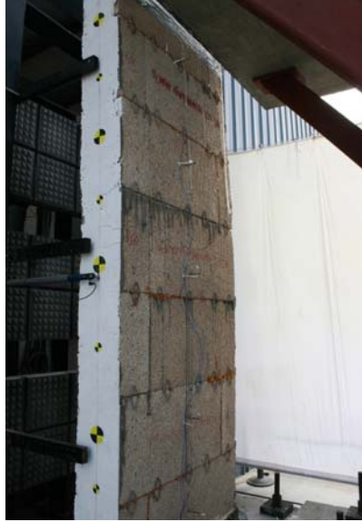
Figure 5.45: Series II frangible panel wall, typical damage
