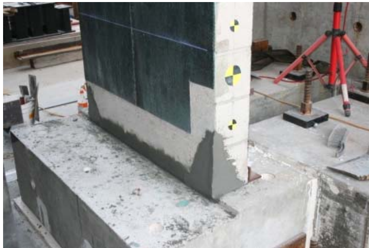
Figure 4.26: Test 6- CMU 3 patched spall areas
