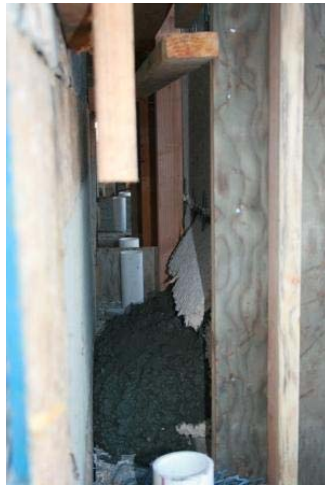
Figure 5.29: Blow out of frangible panel
