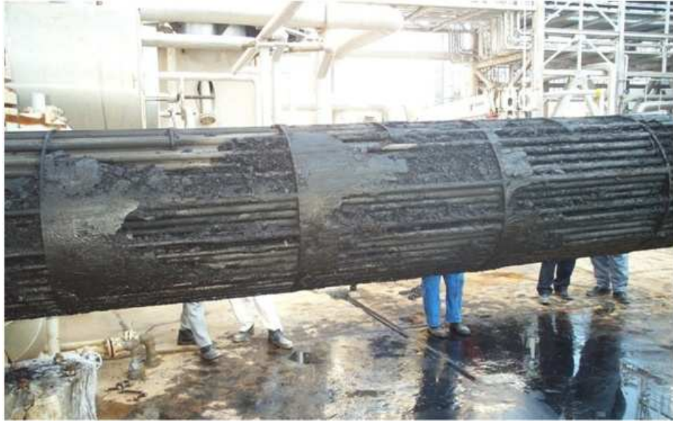
Figure 1.8: Fouled Heat Exchanger Tube Bundles [Ibr12]
