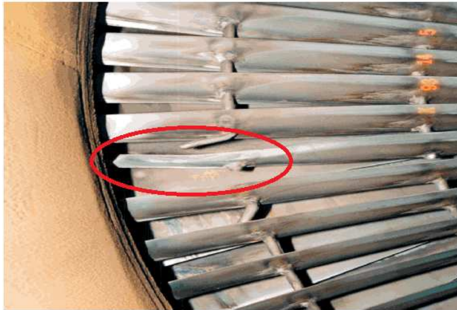
Figure 1.6: Turbine Blade Damage from Wet Steam (Source: PTG Advisers, Inc.)
