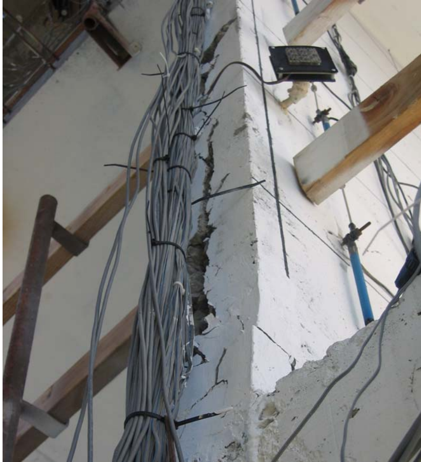
Figure 5.22. Lap-splice failure at bottom of the second story at damage state 4
