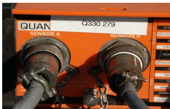
Figure 3.2. Quanterra Q330 instrumented in the tests
