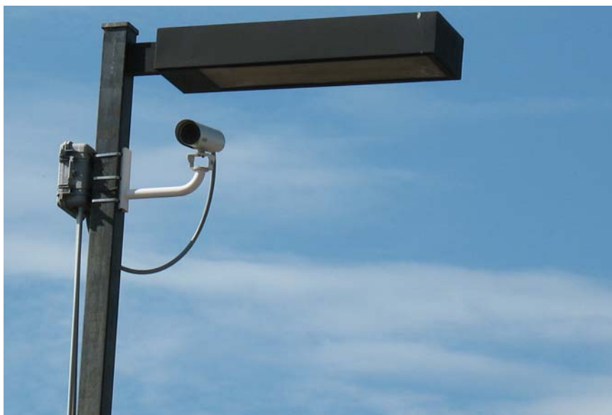
Figure 6.9. Sony XCD-X710CR digital color camera installed in the monitoring system
