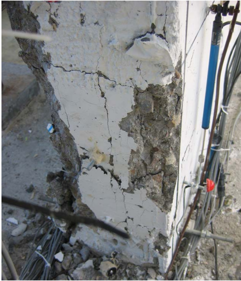
Figure 5.21. Observed damage at bottom of the first story at damage state 4
