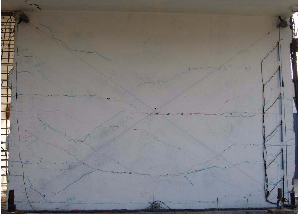
Fig. 6.12 Observed cracks at the first story of the web wall at damage state S4
