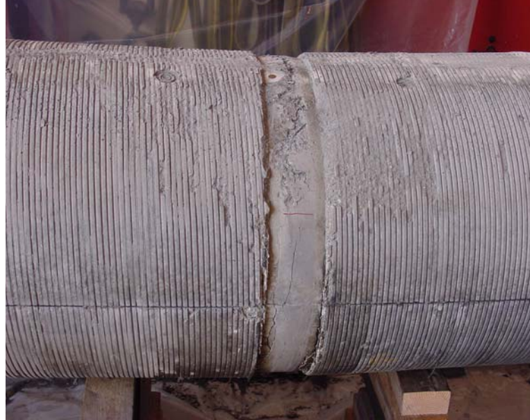
Fig. 5.23 Damage in the concrete core at the splice location
