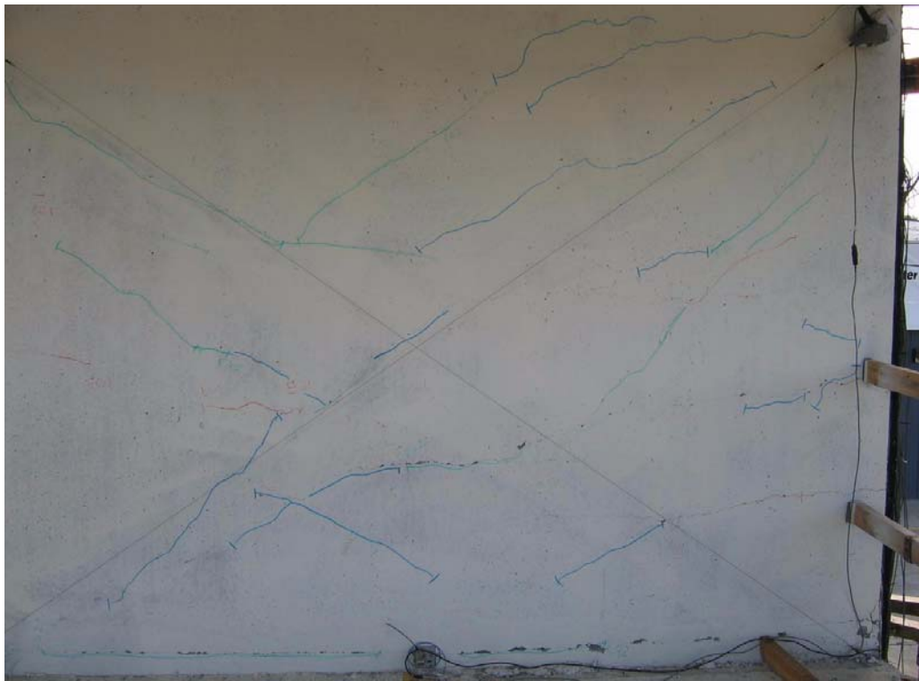
Fig. 6.13 Observed cracks at the second story of the web wall at damage state S4
