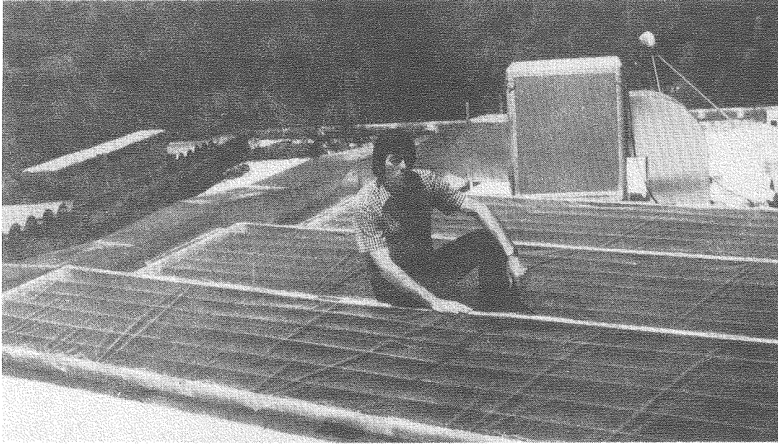
Collector system during active mode.
