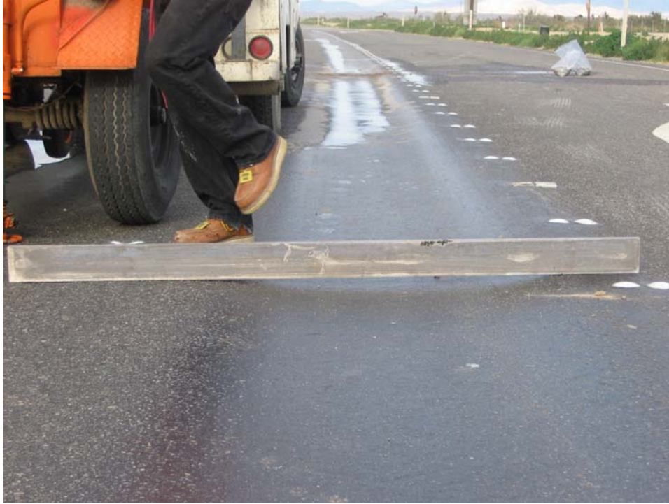
Figure 10. Station 616+21, facing north—note rutting and flushing.
