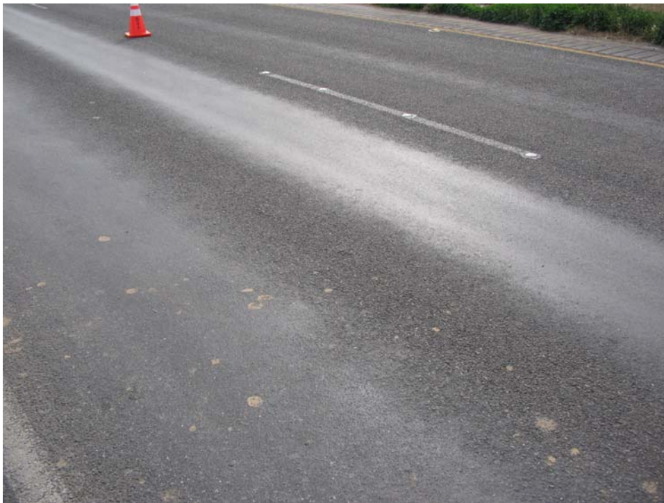
Figure 11. Station 617+60, facing south—clear evidence of flushing in #2 lane.
