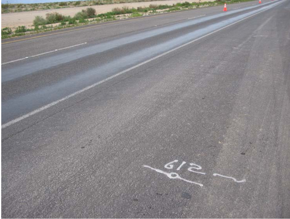
Figure 8. Station 612, facing north—flushing evident in #2 lane.
