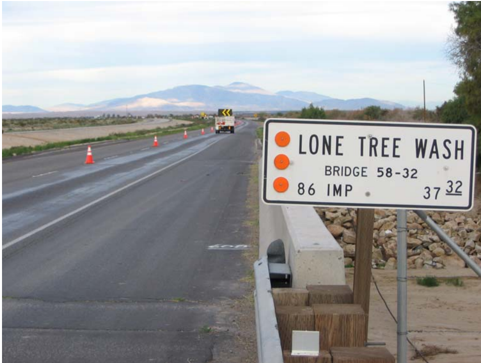
Figure 6. Station 608 (PM 37.3), facing north—flushing evident in #2 lane.
