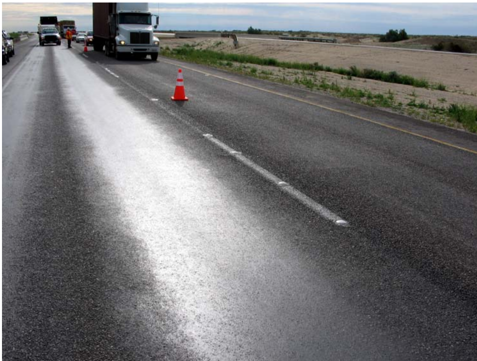
Figure 7. Station 610+40, facing south—flushing evident in #2 lane.
