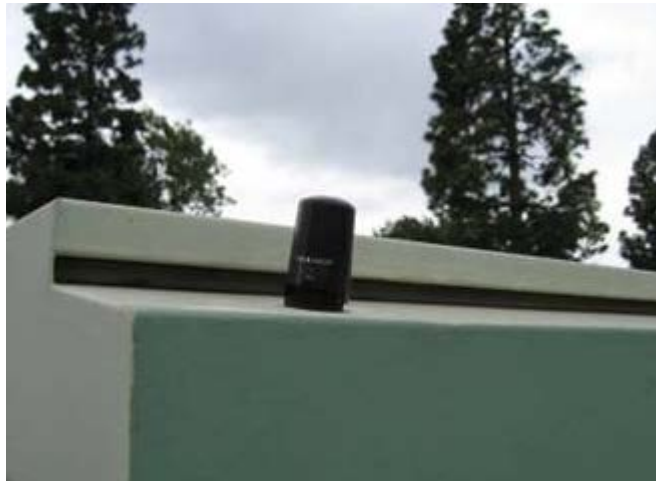
Figure 4-16: Typical WLAN Client Antenna Installation
