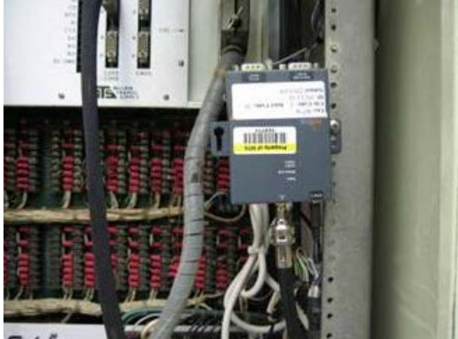
Figure 4-15: Typical WLAN Client Intersection Cabinet Installation
