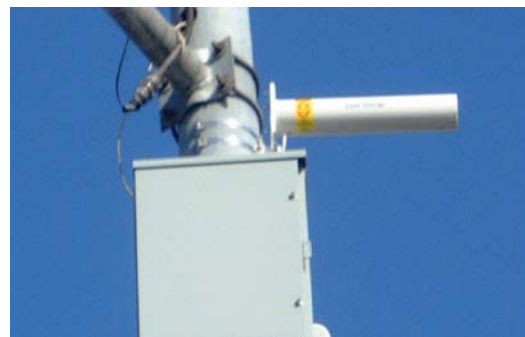
WLAN antenna and equipment mounted at intersection (Photo credit: Steve Gota, LACMTA)
