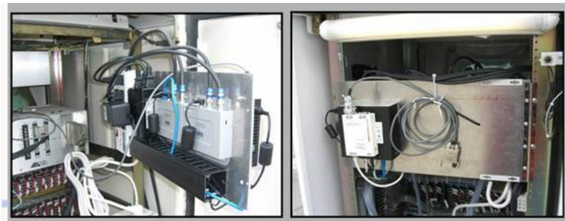
Figure 4-14: Front and Rear Views of Bridge/AP Intersection Panel
