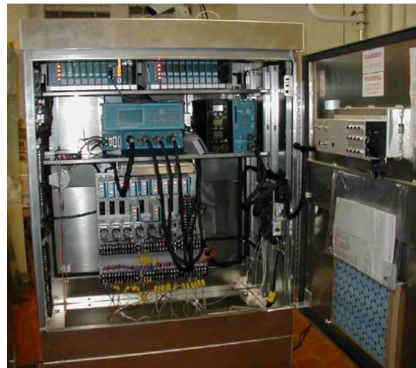
The traffic controller cabinet shown above includes a NEMA Econolite ASC/2 controller. Photo Credit: Peter Koonce
