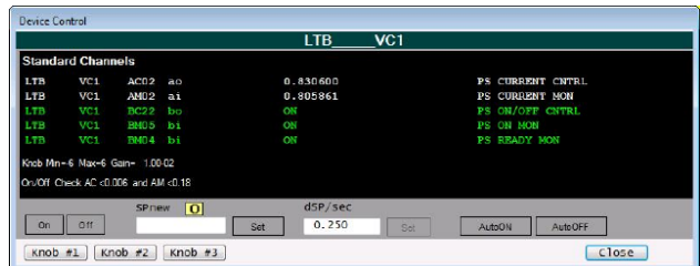
Fig.5. MPS Control Panel
