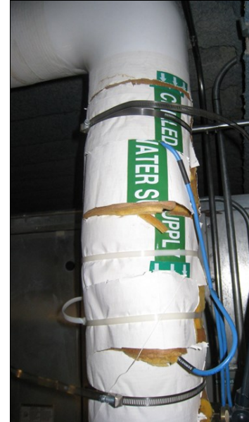
Figure 2.2.1-5d: Chilled water flow and temperature metering
