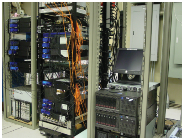
Figure 5.5: PAPER’s 128-input correlator (shown) follows the packetized frequency–cross-multiply (FX) architecture developed by the Center for Astronomy Signal Processing and Electronics Research (CASPER). Shown are 16 ROACH F-engines (left) and 2 dual-GPU box X-engines (right). The first-generation BAOBAB correlator will modify the 64-input, 100-MHz PAPER correlator to become a 32-input, 300-MHz correlator. It will employ eight ROACH boards for spectral processing and four dual-GPU boxes for cross-multiplication. A 10-GbE switch is used to route data between boards.
