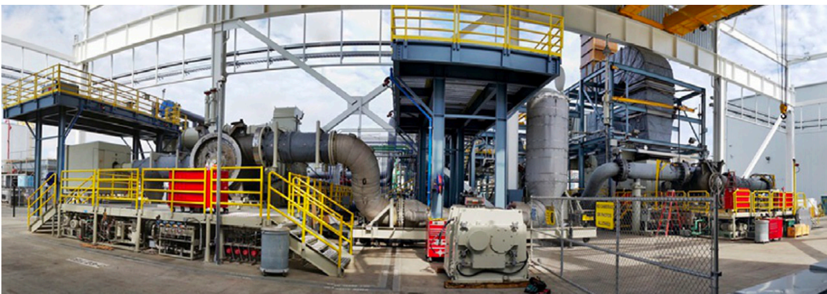
Figure 1.2. Gas compressor test facility (GCTF) at Solar Turbines Incorporated. [13]
