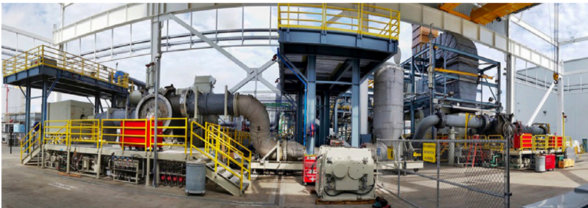
Figure 1. Gas Compressor Test Facility (GCTF) at Solar Turbines Incorporated [13].
