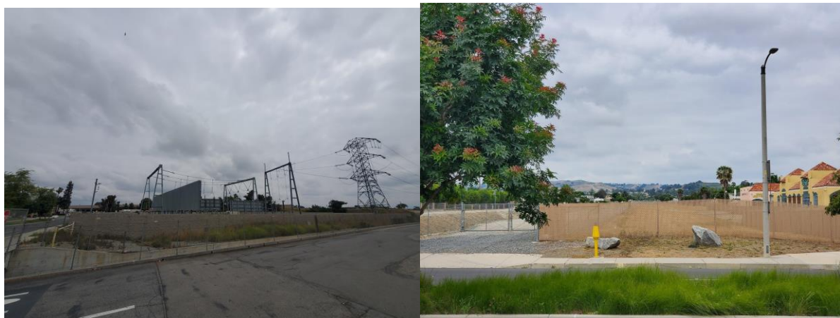
Figure 7: Photos by author, June 2023, from the same location on Pipeline Avenue in Chino Hills. The image on the left shows the substation where the TRTP power lines plunge below ground right at the border between Chino and Chino Hills; the photograph on the right shows the path of now undeveloped land that was previously a site of several TRTP power lines. The former Ryen residence is located in the hills visible on the end of this path, roughly under the large palm tree in the foreground on the middle right.
