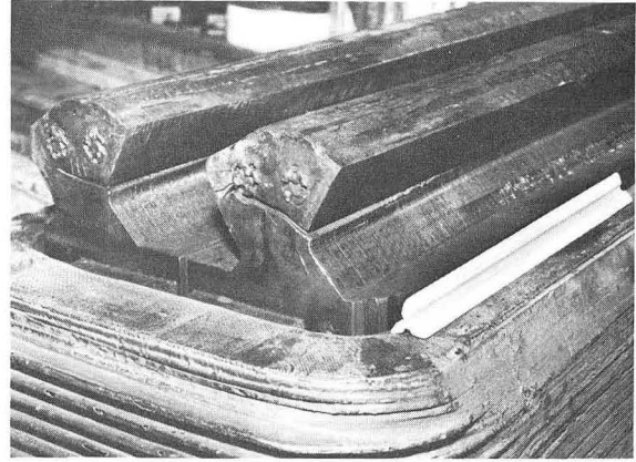
Fig. 2 Extent of Dovetail Cracks
