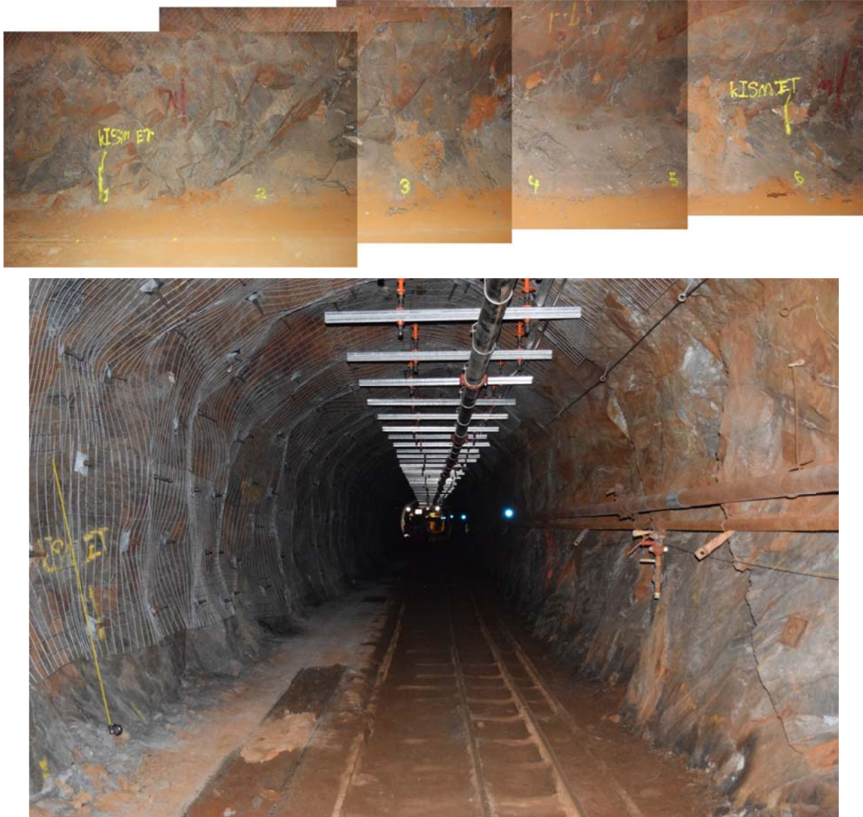
Figure 2.10. Upper image: Composite photo of site taken on May 21, 2015 spanning approximately 60 ft (18.3 m) along the east rib of the West Access Drift. Lower image: Photo taken in February 2016 showing new ground support consisting of rock bolts and wire mesh. (For reference, the yellow kISMET spray paint on right-hand side of upper image is the same as that in left-hand side of lower image.).
