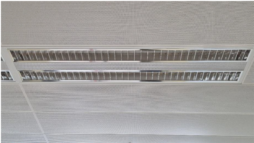
Fig. 2. Recessed luminaire with fluorescent lamp in room 518.
