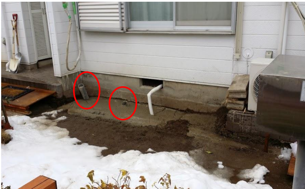
Figure 14: Grouting pipes installed for compaction grouting outside a private residence in Japan
