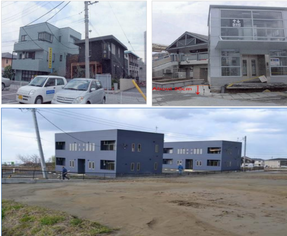
Figure 5: Large settlements and tilting of building due to liquefaction effect in Japan (Ashford et al. 2011)
