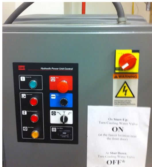
Figure 97. Main hydraulic pump
