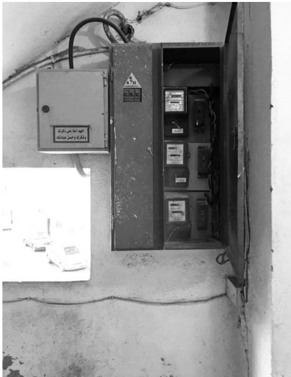
Figure 3-5. Image of electricity meter boxes installed by the Jordanian Electric Power Company. Photograph by author, August 2019
