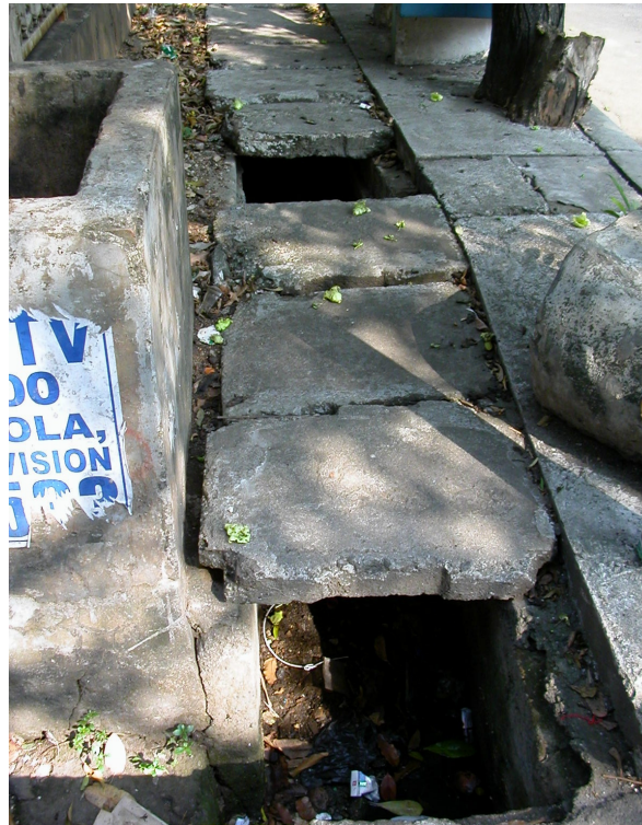
Figure 14: Broken culvert covers create dangerous sidewalk conditions in Central Jakarta
