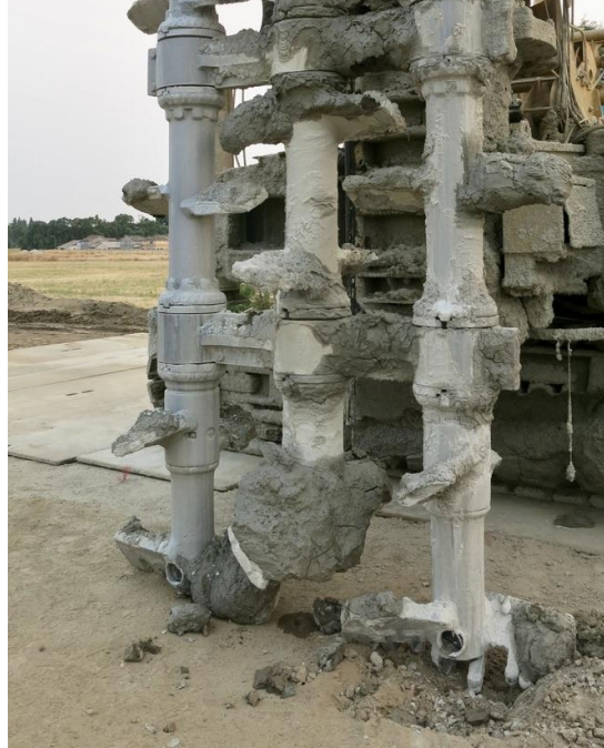
Slurry injector for fixing the levee in place. Northern levee. August 7th, 2018
