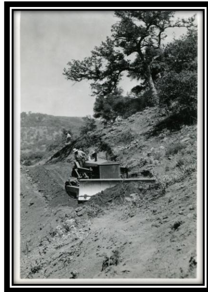
Photograph 2. Bulldozer grading one of the new roads on the Santa Ysabel Indian Reservation (c. 1938). From the records of the Bureau of Indian Affairs, Record Group 75, National Archives Pacific Region (Laguna Niguel).
