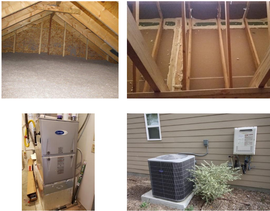
Figure 11. Basic cluster (top) and HVAC cluster (bottom) example project images. Attic blown cellulose insulation (top left), attic framing air sealing (top right), gas furnace (bottom left) and split heat pump (bottom left). (Image credit: Building America Solution Center, Image Gallery).
