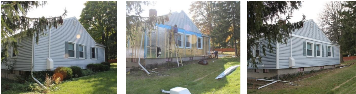
Figure 14. Superinsulation cluster project images. Before (left), during (bottom) and after (right) exterior wall insulation upgrade. (Image credit: Jon Harrod of Snug Planet).
