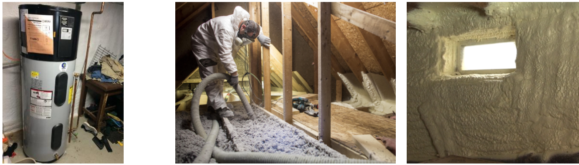
Figure 15. Electrification with PV cluster project images. Post-retrofit exterior images including solar PV (top left and middle), Tesla battery pack (top right), heat pump water heater (bottom left), cellulose attic insulation (bottom middle) and closed cell spray foam basement wall insulation (bottom right). (Image credit: Zero Energy Now (ZEN) Program, VT).
