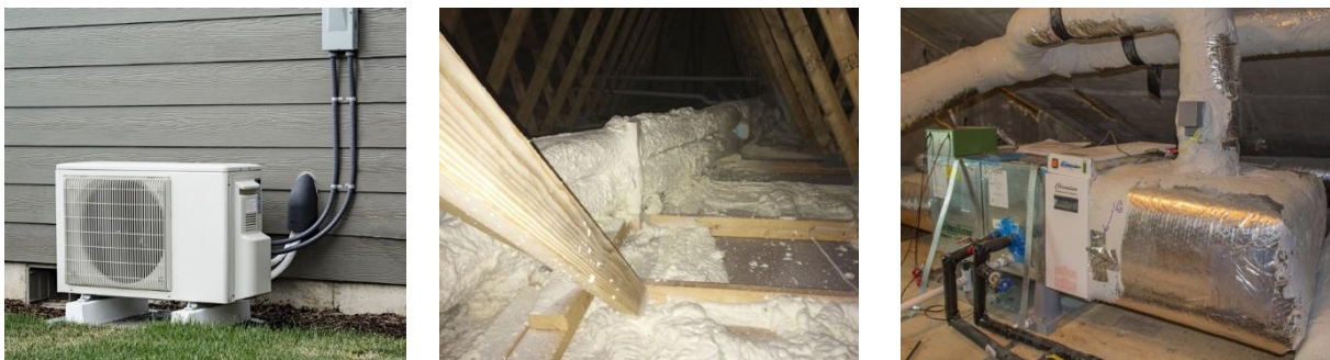
Figure 12. Advanced HVAC cluster images. Heat pump outdoor unit (left), encapsulated ducts using spray foam (middle), and air-to-water heat pump with advanced filtration and outdoor air intake (right). (Image credit: Building America Solution Center, Image Gallery).
