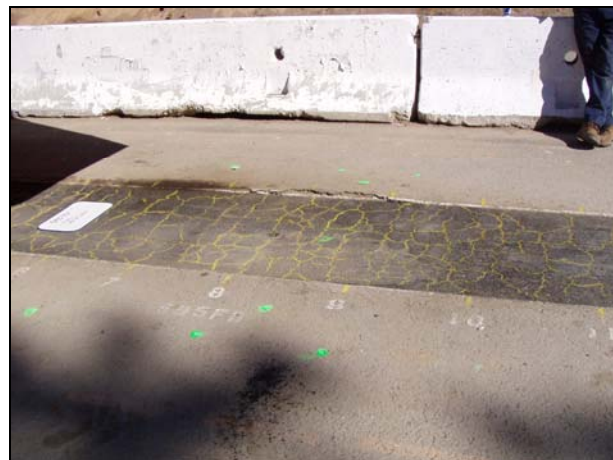
(b) Extensive fatigue of Section 595FD at end of test
