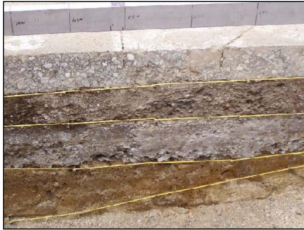
Figure 4.28: Test pit on Section 594FD after HVS trafficking.
