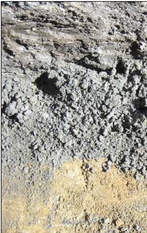
(a) Grey colored material found below the base layer on the HVS lane
