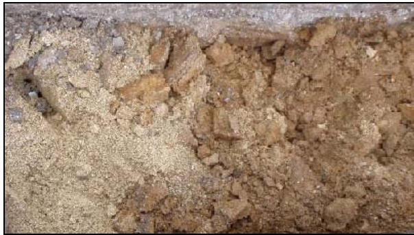
Figure 4.32: Two materials in subgrade on Section 595FD.
